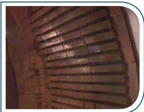
White iron lined impact wall
