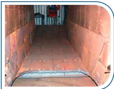
Load out chute protected with NiHard liners
