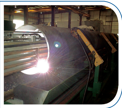
The circumferential overlay process and oscillated weld bead, produce an industry leading end product
